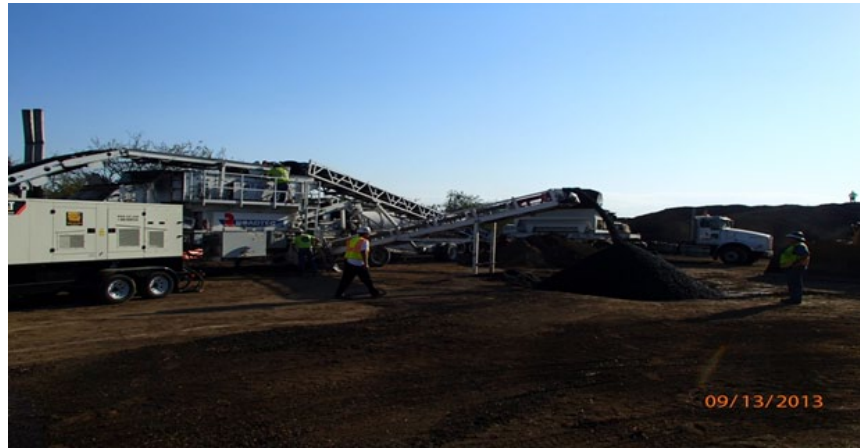
Figure 8. Cold Central Plant Operation for Ord Ferry Road FDR-C Project.
