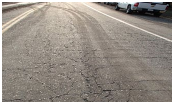
Figure 1. Existing Pavement Condition at the Ord Ferry Road before Construction
